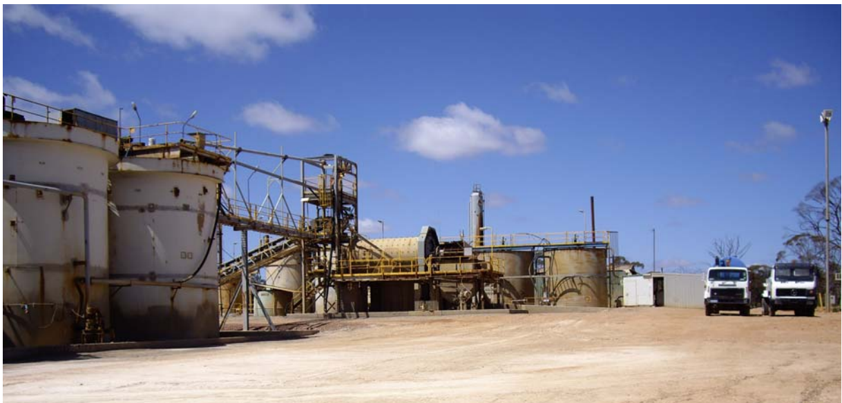
Figure 2. Ball mill and leaching tanks at Nimbus processing plant (photo courtesy: Polymetals Group Pty Ltd).
